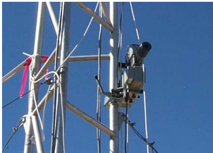
Figure 5. Ultraviolet Ion Collectors (UVIC) mounted on a 6-m tower (Photo by Sam Chang, ARL).
